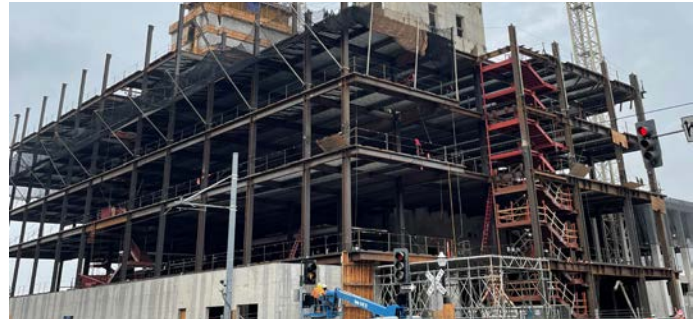
The new Sacramento County Courthouse under construction in mid-November 2021. The 17-story, 53-courtroom courthouse is located in Downtown Sacramento on the block bordering H and G streets and 5th and 6th streets behind the federal Robert Matsui United States Courthouse. The new courthouse will replace the existing courthouse at 720 9th Street and will cost nearly $500 million to build. Located on the southeast corner of The Railyards, the Sacramento County Courthouse is scheduled to open by year-end 2023.
