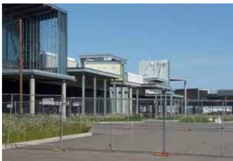
The half-built Elk Grove Promenade project sits like a ghost town at the Highway 99 and Grant Line Road exit in Elk Grove, but this may not be the case for much longer. Owner GGP is about to emerge from bankruptcy. One possible scenario is that GGP will be split into two entities; one that would keep the majority of the Chicago-based REIT's performing retail holdings and one that would be charged with the disposition of troubled assets like the Promenade.
